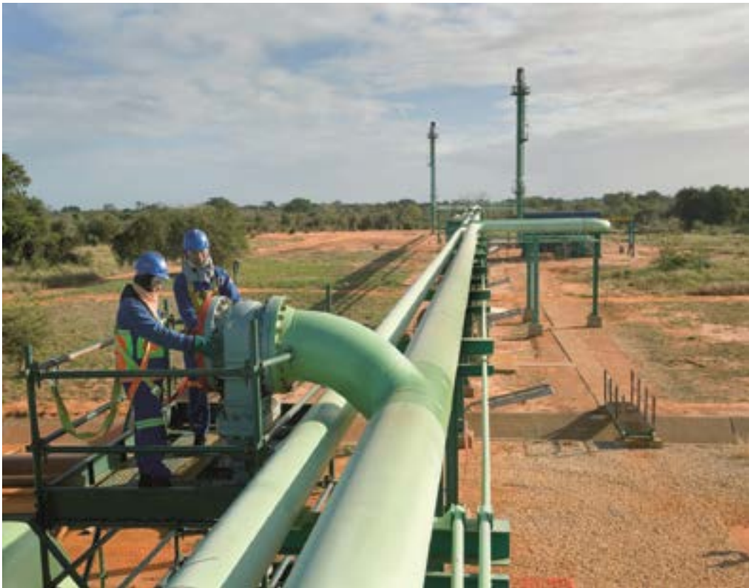
SASOL gas pipeline in Temane, Mozambique
